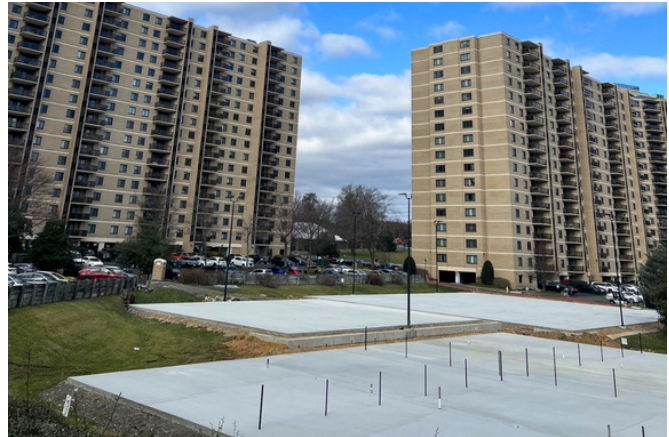
The Outdoor Courts concrete work and Bldg 3 Completed Balcony Projects. Photo by Brianna Hawkins
