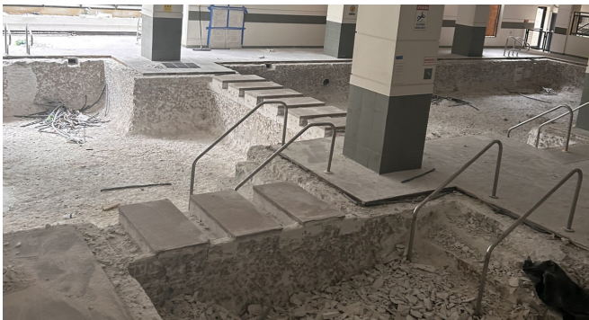
CWC completed concrete work. The Indoor Pool is anticipated to open to residents and swimmers in October!
